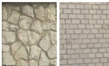
Stone/dressing that does not match the vernacular: (clockwise from top left) jumping stones; rock faced; white limestone; un-coursed random rubble
